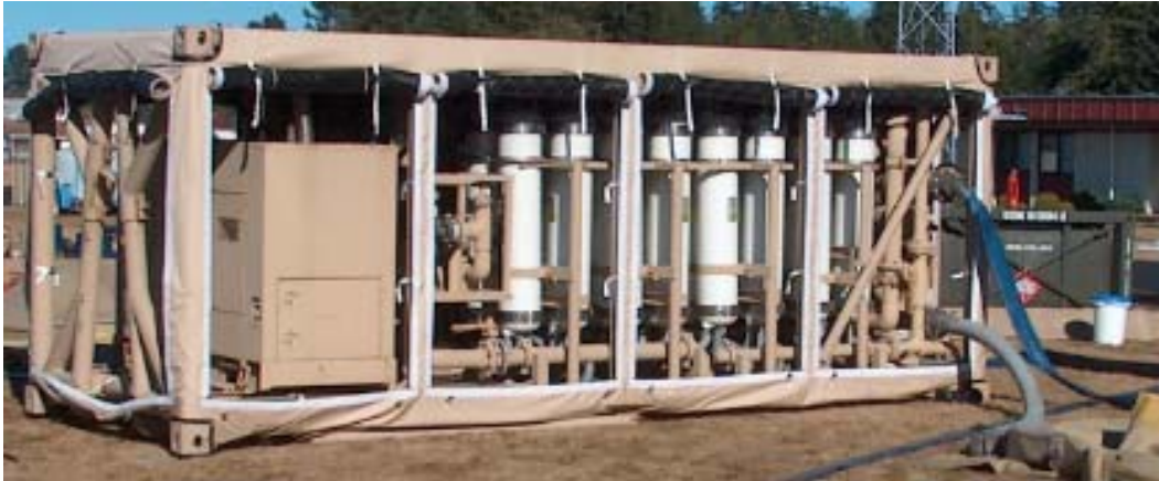
Figure 5-4. – Photo of the UF skid.
