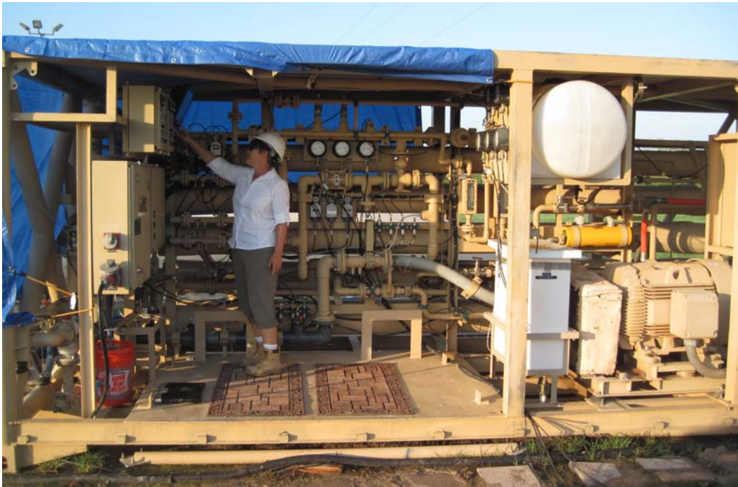
Figure 5-5. – RO skid and control center.
