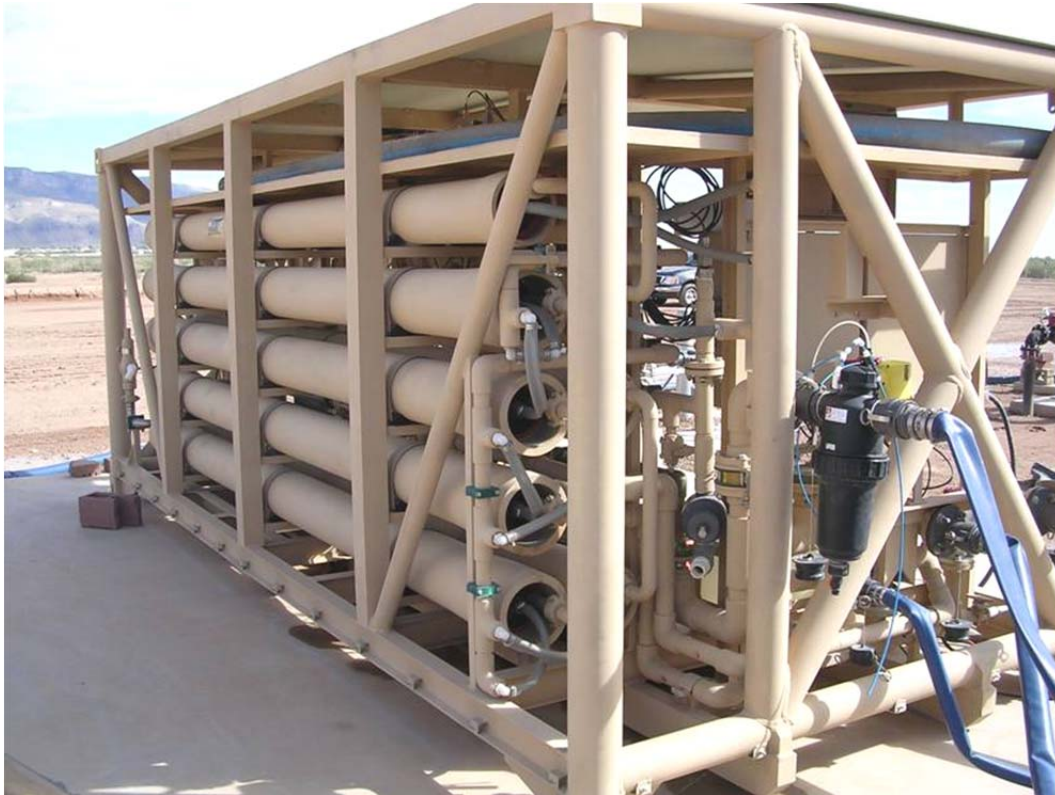
Figure 5-6. – RO skid showing RO vessels.
